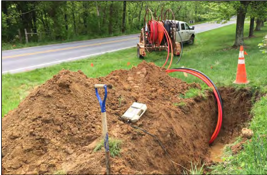
Figure 16. PE conduit being dispensed from the top of a 3-way segmented reel to minimize the bend radius; conduit is installed using horizontal directional drilling (HDD)
